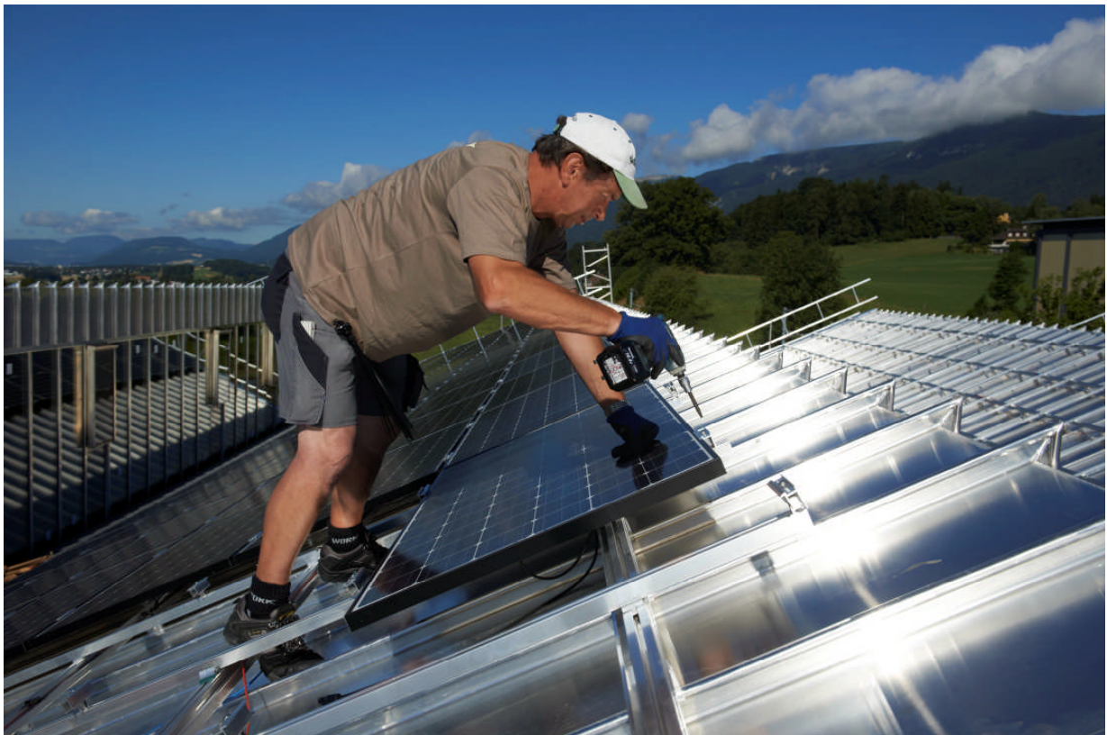
Figure 1: Mounting procedure on the roof of Truninger AG's production site in Switzerland
