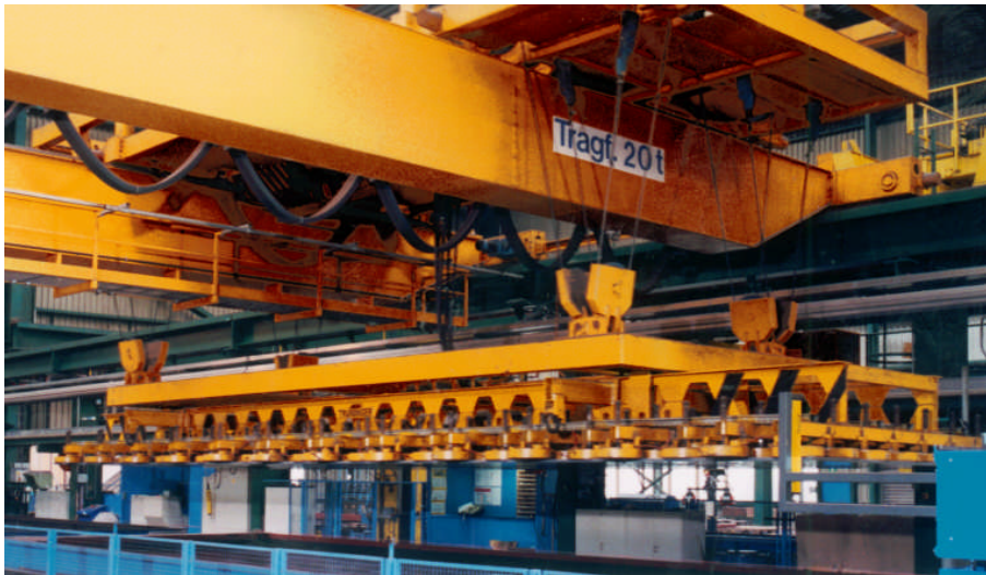
Figure 2: Special spreader beam for placing large sheets on the table; off-cuts and scrap parts get cleared away in one lift
